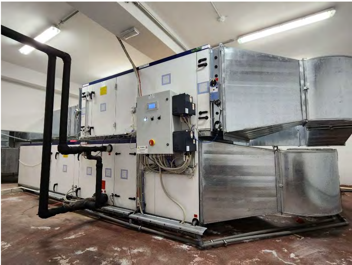
Figure 4.21 – Air Handling Unit (AHU)
