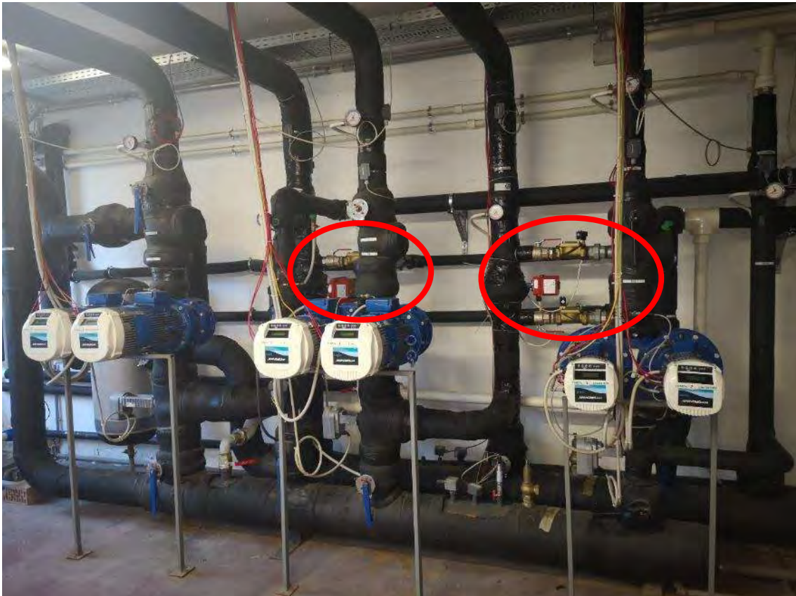
Figure 4.21 – Hydraulic Distribution System of ICSTM
