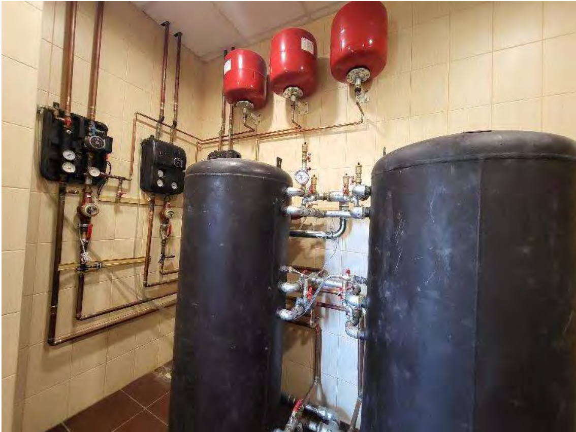
Figure 5.1 – Space arranged for the new solar thermal installation
