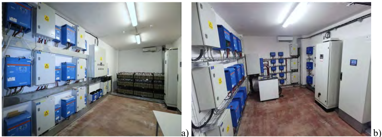
Figure 6.2 – Microgrid System: a) initial; b) current, after 2021
