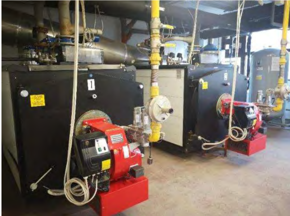
Figura Error! No text of specified style in document..6 - Fotografie cazane centrala termica ICSTM
