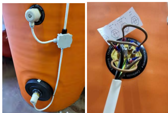
Figure 6.5 – Installation of resistances on the boiler
