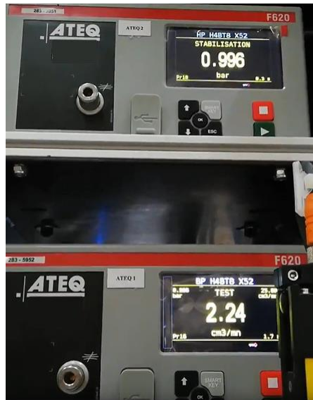
Fig. 14.3 - High pressure test/Low pressure stabilization
