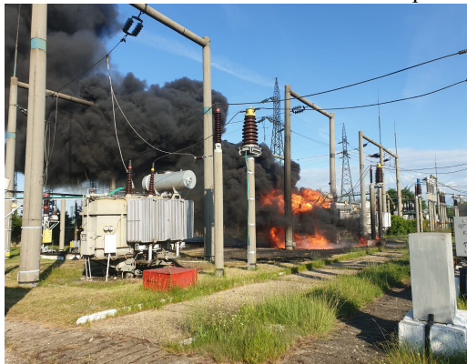
Fig. 10. Recent fire at a transformer in Adjud, Vrancea, Romania
