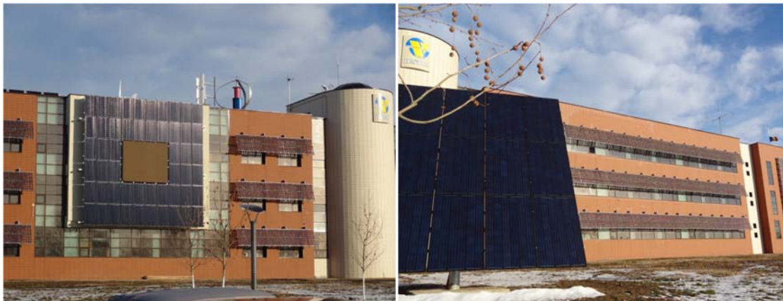
The pilot self-consumption installation
