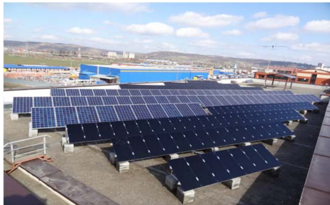
Photovoltaic system installed on the roof of our Institute building-ICSTM
